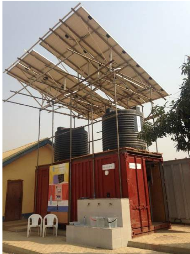
Solar Powered Drinking Water Station PVWater International Dutse/Abuja
