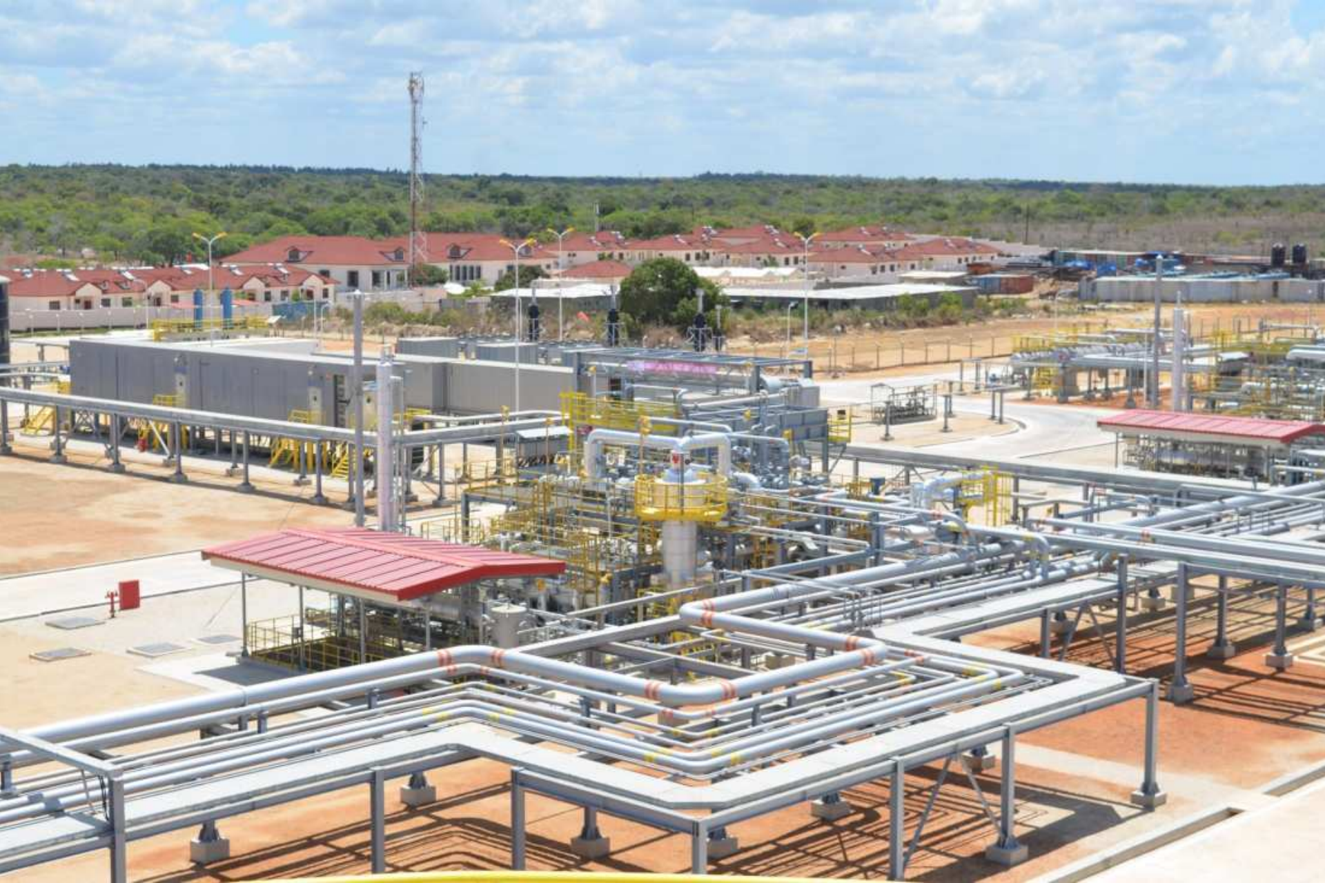
Gas processing facility in Madimba – Mtwara
